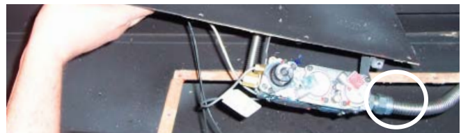
Gas Inlet Line
