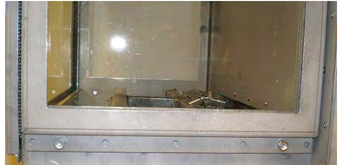
Bottom of Glass Door Frame
